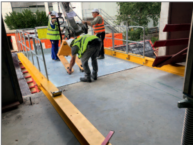
The aluminium props are simply folded up and fixed work platform is clearly visible
